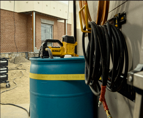
Able to transfer a 60% water/40% propylene glycol mixture
